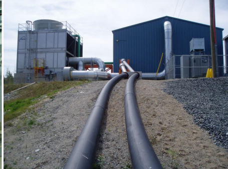
Refrigeration plant exterior (source: Mining Magazine, 2007).
