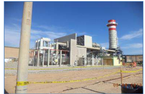
Turbina a gas (TG2)
