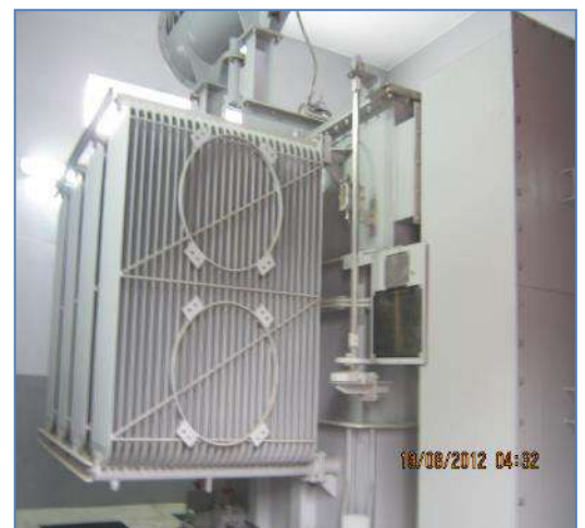
Transformador Principal 17/20 MVA 13,8/22,9 kV
