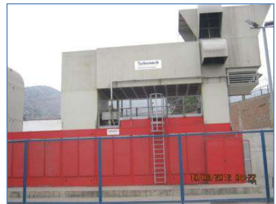
Turbina a Gas
