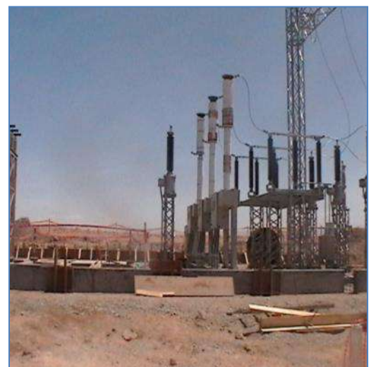
S.E. Central Panamericana Solar (23/138 kV)
